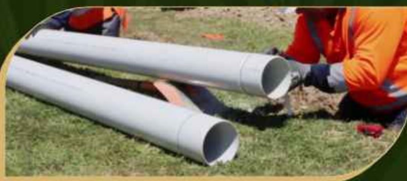
Water Pipe Line
